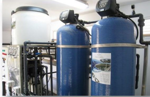
Figure 12: Pre-filtration unit in Zbeidat desalination plant
