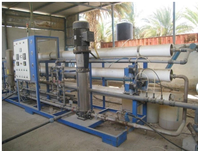
Figure 21: PARC R.O Unit
