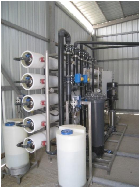
Figure 23: R.O unit at COPSCO desalination plant
