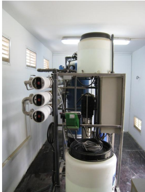
Figure 14: Anti-scalant unit in Zbeidat desalination plant
