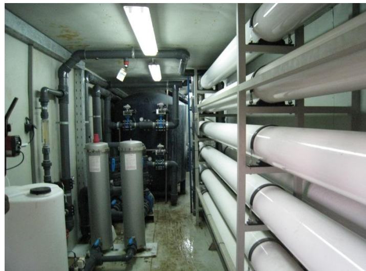
Figure 18: Pre-filtration unit –Marj Na'jeh plant
