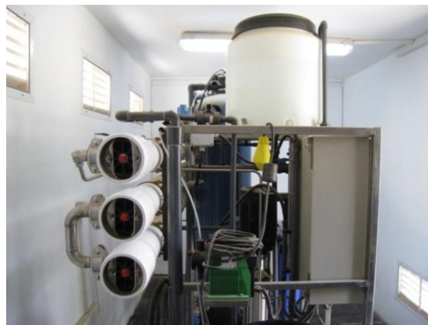
Figure 13: R.O unit in Zbeidat desalination plant
