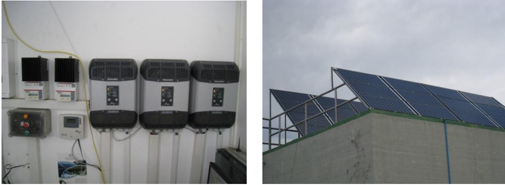
Figure 15: PV energy supply system in Zbeidat desalination plant
