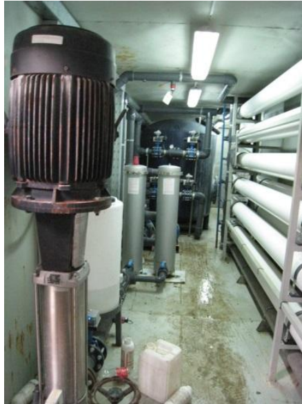
Figure 19: R.O unit –Marj Na'jeh plant
